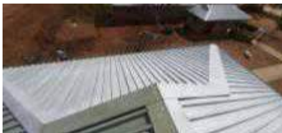
Cool Roof Surface Project supported Early Childhood Development Centre and primary school at Air Force base Makhado
